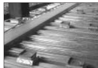
Trenchduct utilized to feed wire and cables to N-R-G-Flor.
